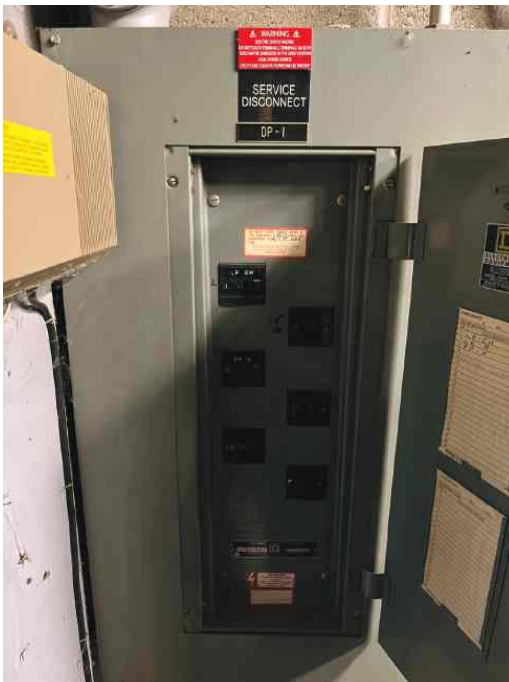
Existing electrical panel
