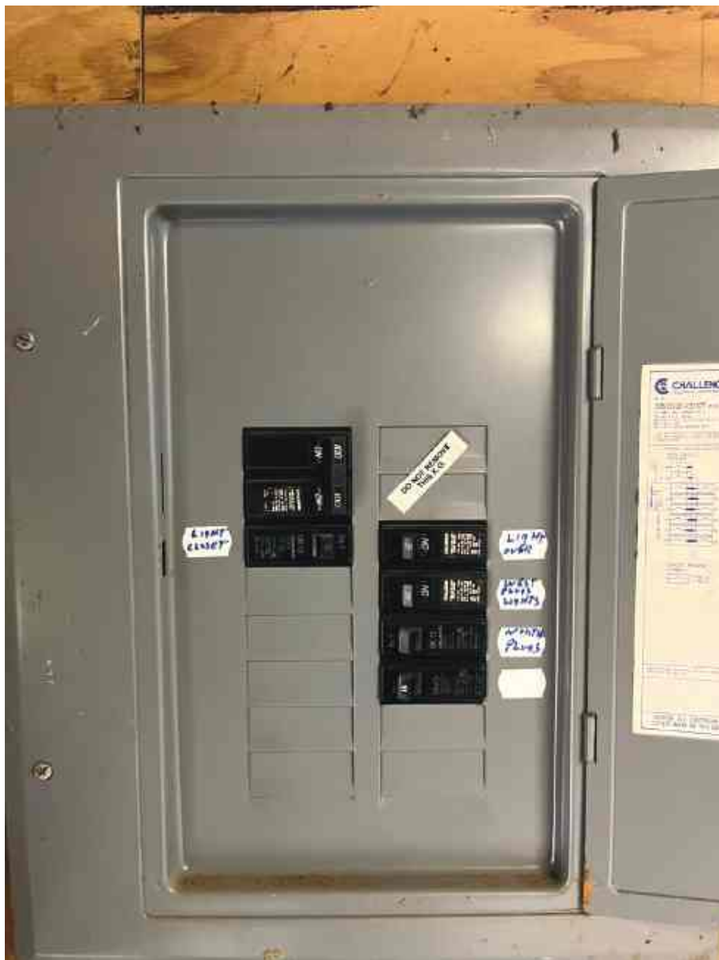
Existing electrical panel
