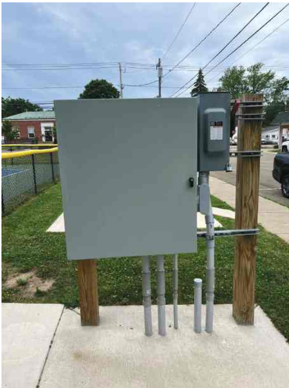
Electrical Panel at Court
