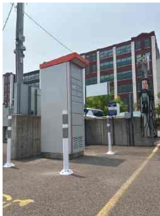
Figure 17: Swobbee unit being tested on the Buffalo Niagara Medical Campus
