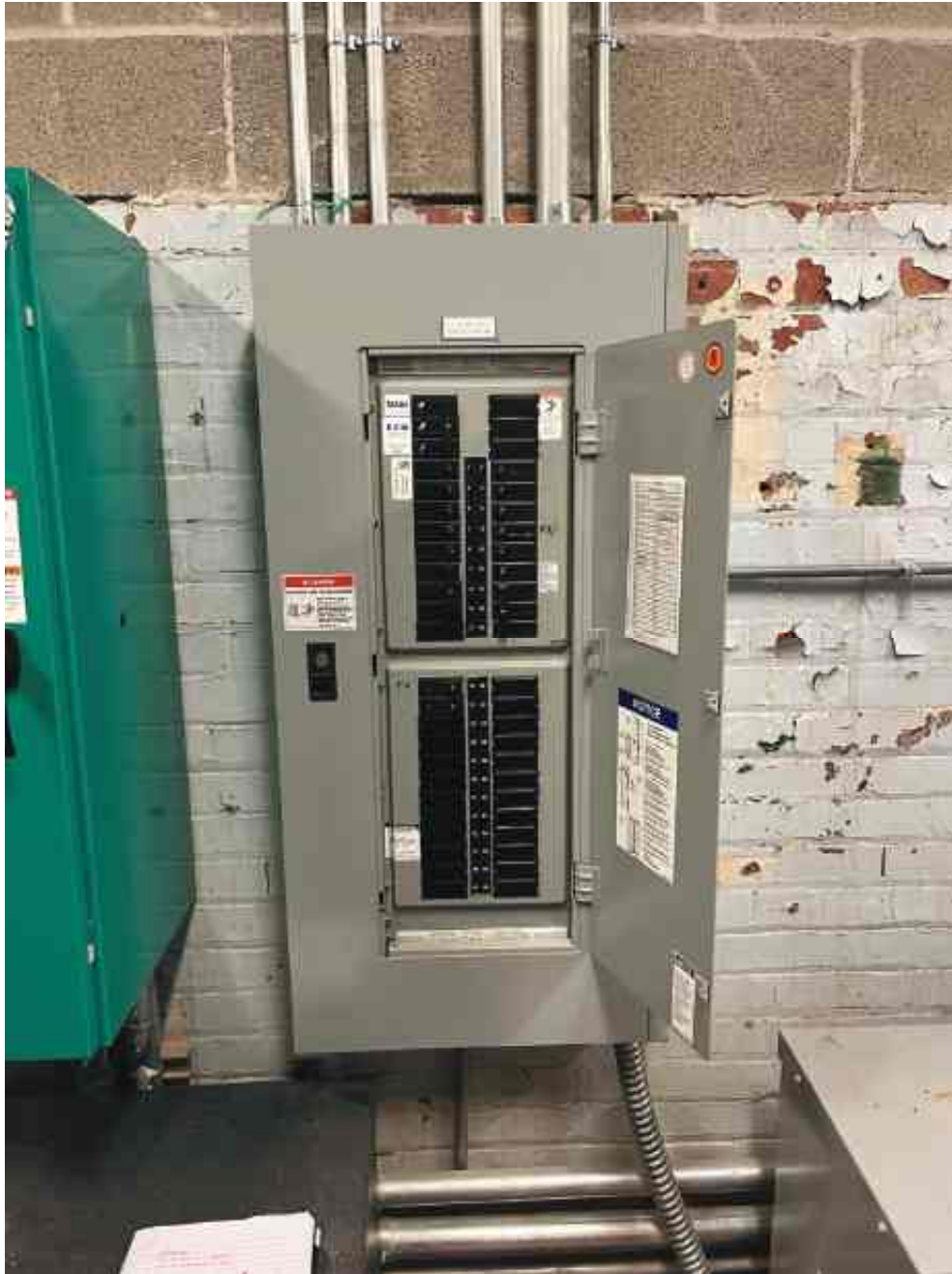
Existing Electrical Panel LV-SB-PP in Main Electrical Room
