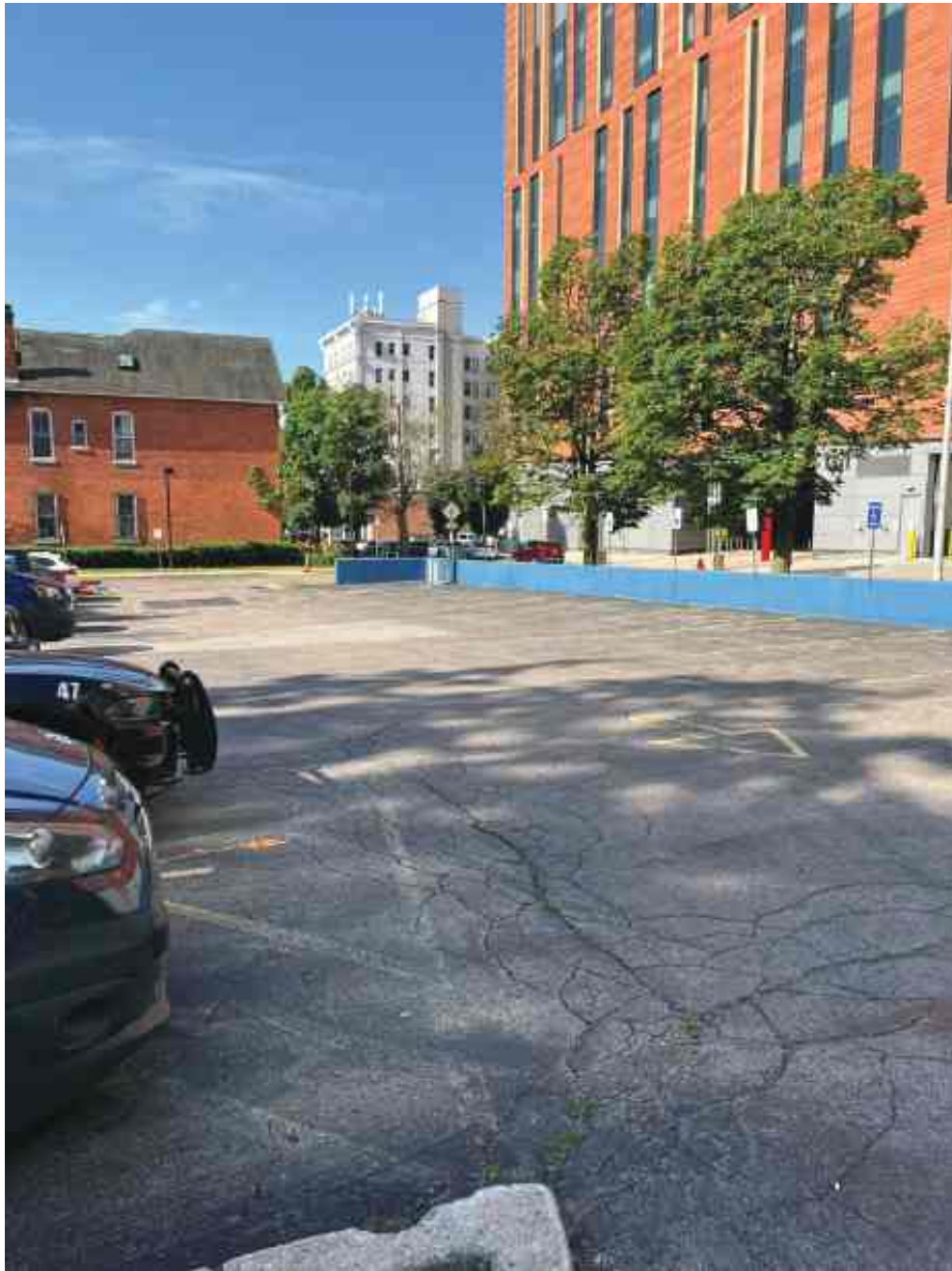
Non-functional EV charger and proposed EV, e-bike charger and locker location
