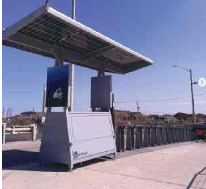
Figure 10: Skyhook 6 Panel Solar charging a bikeshare system
