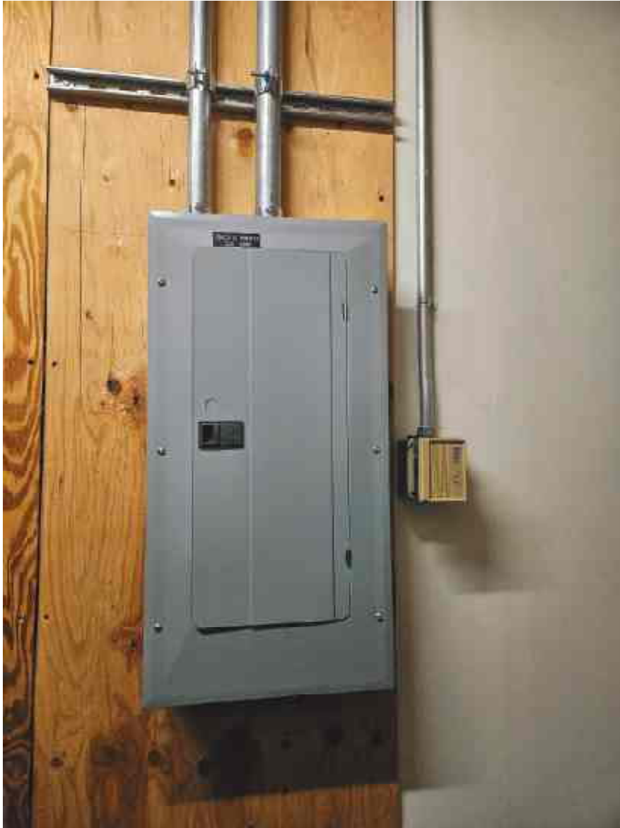
Electrical Vehicle Sub Panel
