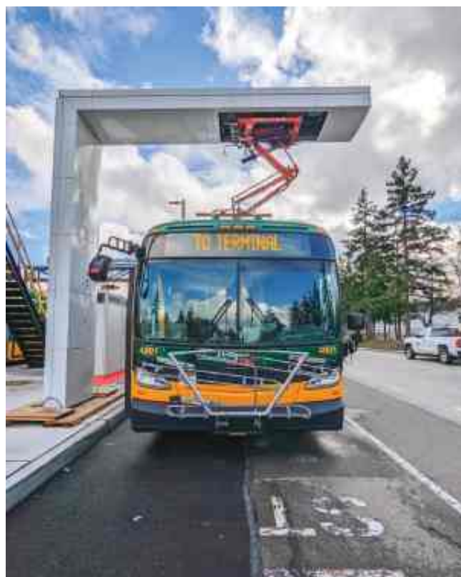
Figure 12: McKinstry mid-route bus charger, King County Washington
