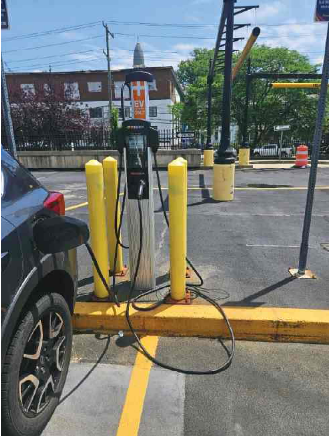
Existing EV Charger
